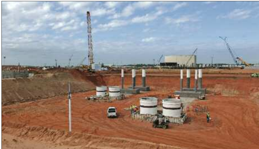
This shot of the Vogtle new construction site, taken on November 3, 2011, shows circulating water system pipes that will connect to Unit 3's turbine building and condenser. (Photo: Southern Company)
